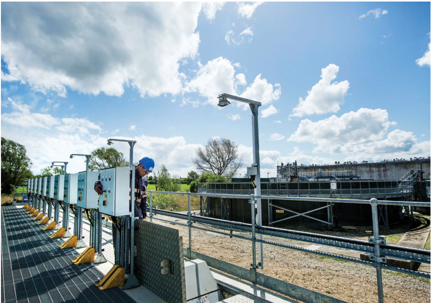
Wedeco Duron UV installation in Chichester, UK.
